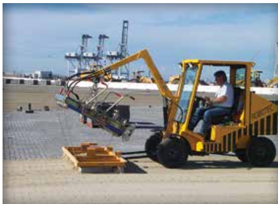
Figure 12. Sweeping jointing sand across the pavers is done after the initial compaction of the concrete pavers.
