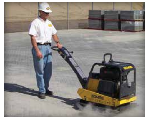
Figure 13. Final compaction should consolidate the sand in the joints of the concrete pavers.
