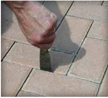
Figure 14. A simple test with a putty knife checks consolidation of the joint sand.
