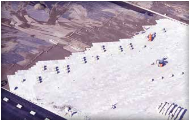
Figure 7. Maintaining an angular laying face that resembles a saw-tooth pattern facilitates installation of paver clusters.
