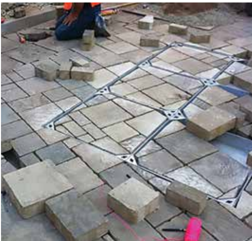
Figure 27. Another example of cutting pavers to accommodate a utility cover set at an acute angle to the paving slab pattern
