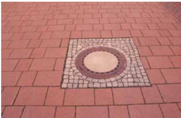
Figure 28. Filling the outside of a utility cover with mortar-set stone paving units
